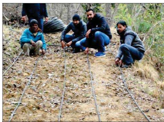
Installed drip irrigation system in Salla Rautela
